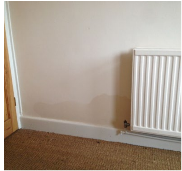
Figure 8 Damp in solid brick wall (from puddle in side passage, courtesy of the AECB Carbonlite Retrofit course)
