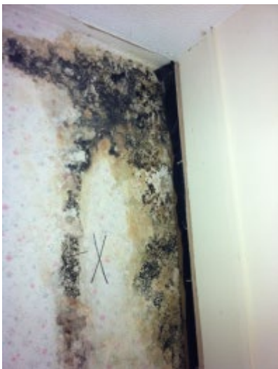
Figure 13 Laminate board installed on timber stud cavity with NO ventilation, poor air barrier and poor external pointing. Black mould was found growing in the narrow space behind, feeding off the wet wallpaper 11 .
