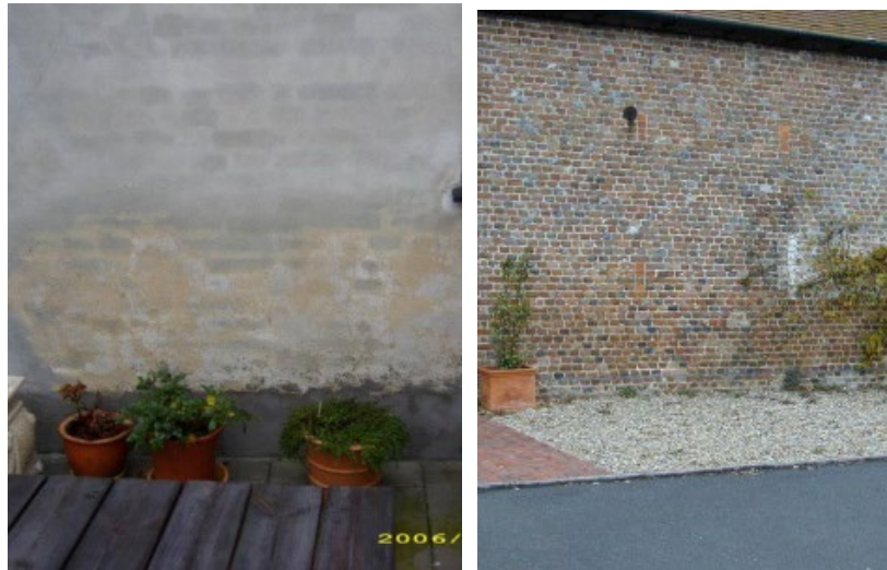
Figure 2 Examples of visible rising damp (courtesy of the AECB Carbonlite Retrofit Course)
