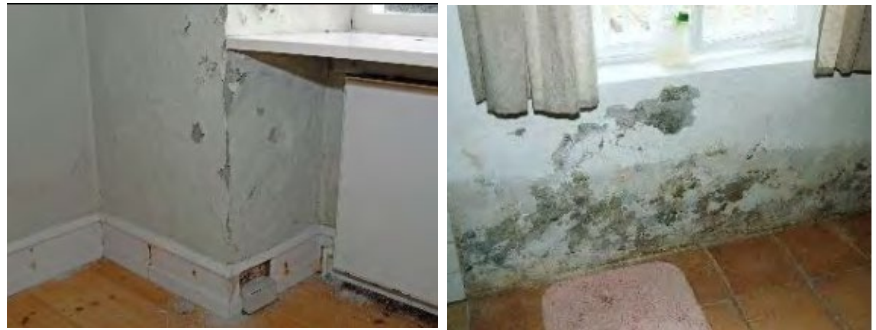
Figure 7 Paint and plaster deterioration (courtesy of Aalborg University)
